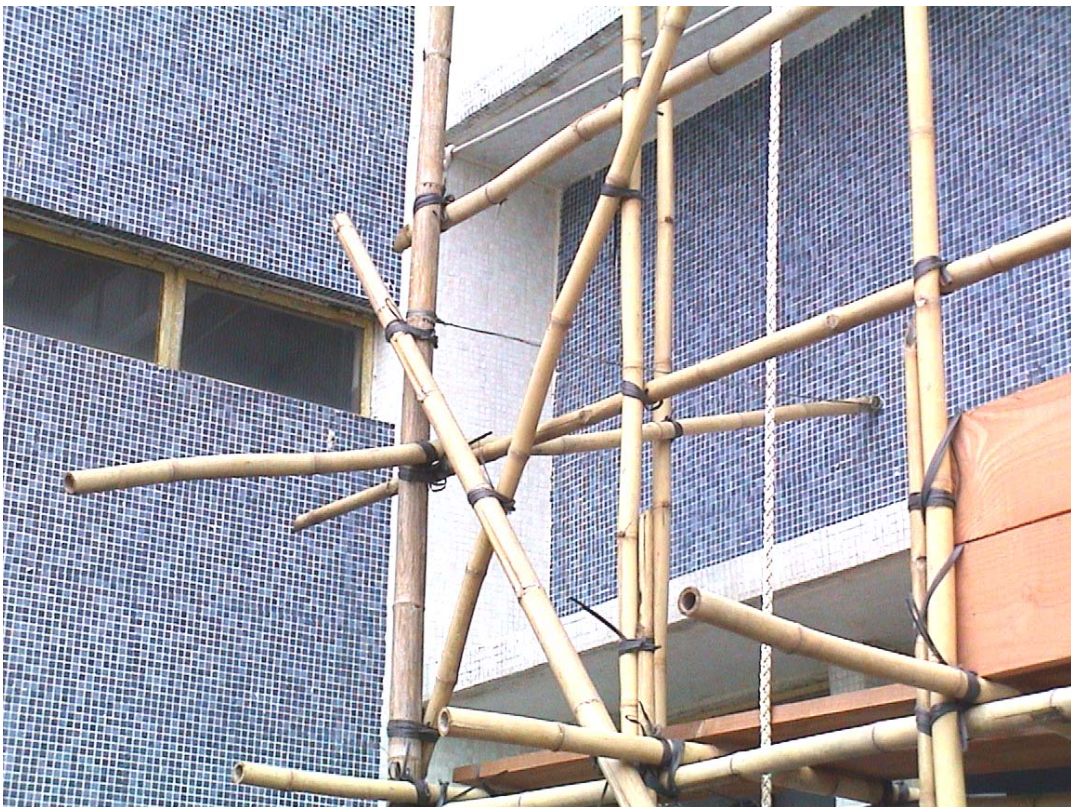
Figure 1.5 Detail of a putlog attaching the post of the outer layer in a DLBS
